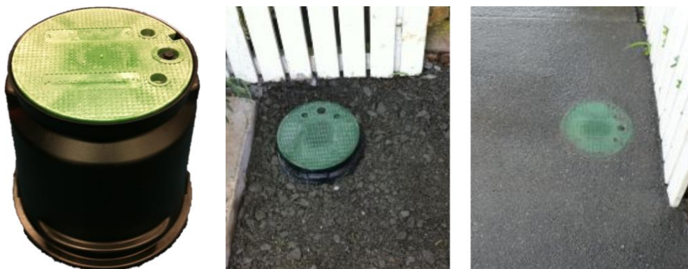
Figure 1. Channell Hand hole at the Premises Boundary
